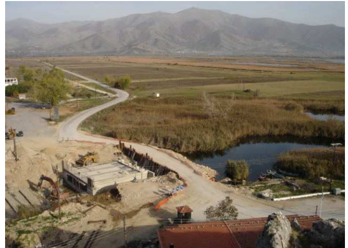
Sluice works (A. Rigas, SPP)
