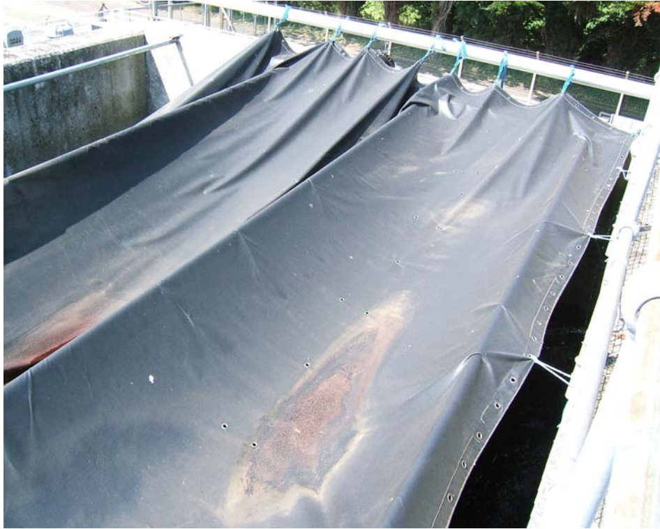
Figure 5.19 Coverage of filters protects from algal growth at Wessex
