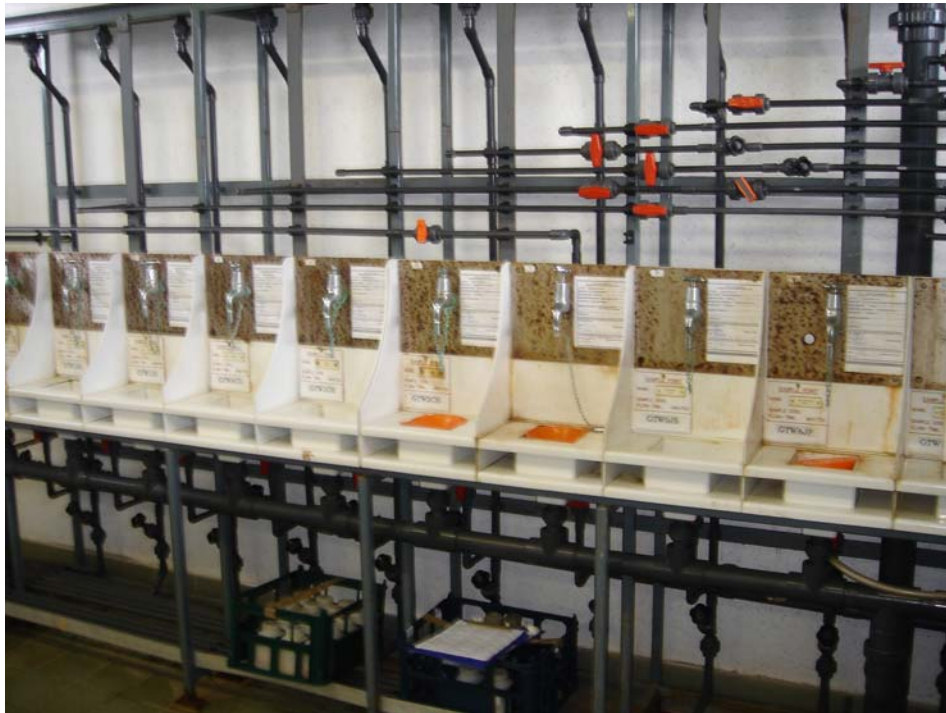
Figure 5.18 Centralized sampling points allow easy access to all unit operations
