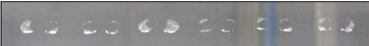
Figure 43 Cracks in glass caused by soldered connectors as visible from the outside face of the product (ACEA et al. 2009)
